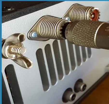
Coax Center Conductor Only—measure noise level
